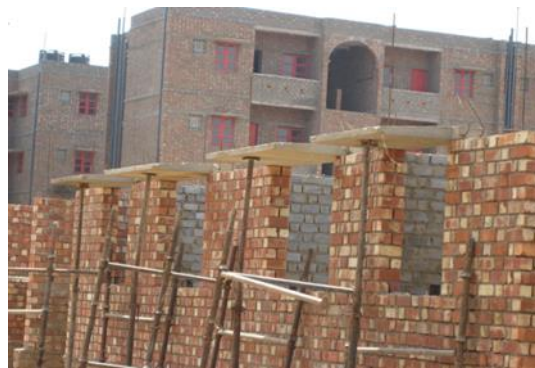
Figure 5. Application of Modular Fly ash bricks in a 4-storied housing at Baprola, New Delhi, India
