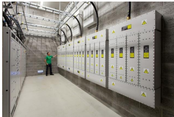
Figure 10. HEMP filters installed in a military bunker protected against the nuclear explosion
