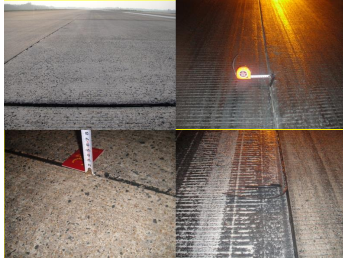
Figure 3. Caulking material damage and dislocation
