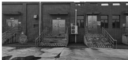
Figure 4. Aboveground transformer and distribution room
