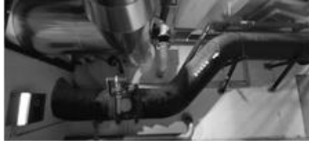
Figure 6. Accidental sewage overrunning pipe
