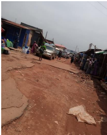
Figure 13. Image of the Derelict Road Network and dilapidated Drainages
